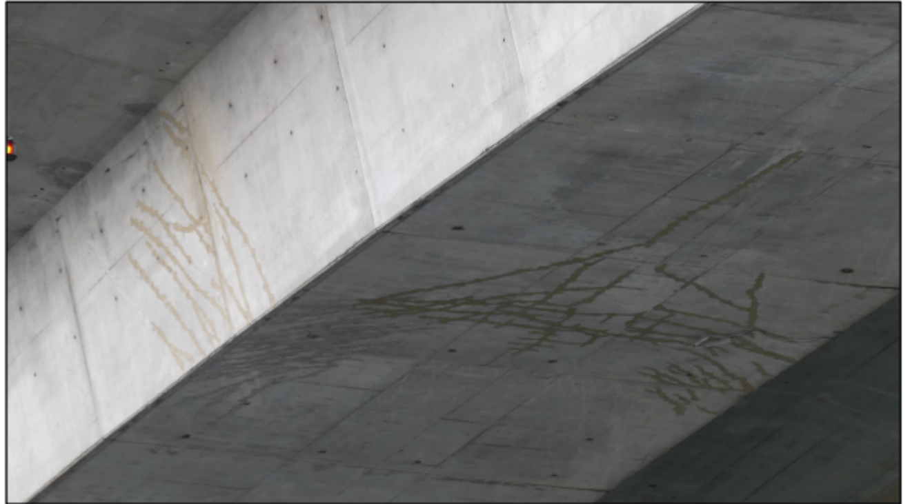
Location P1 Defect J38SE:
